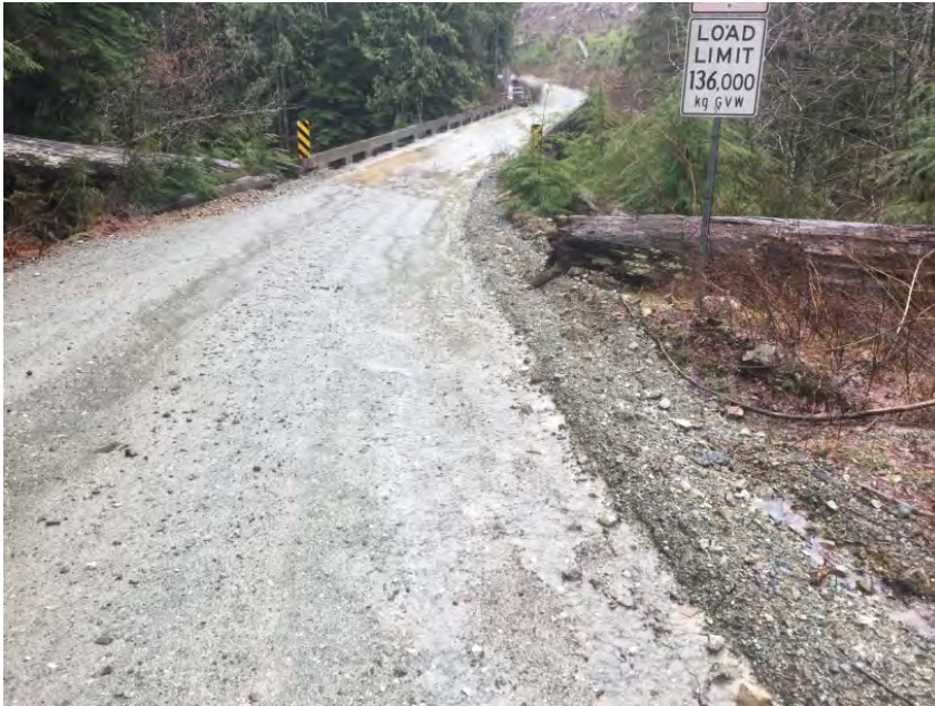
Grader berm directing surface water onto bridge deck
