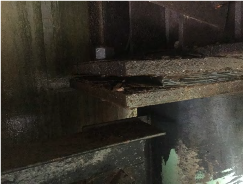
Minor delaminating of DS left bank bearing plates
