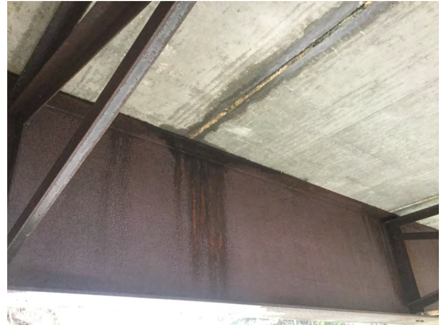
Indication of water leaking through random deck joints
