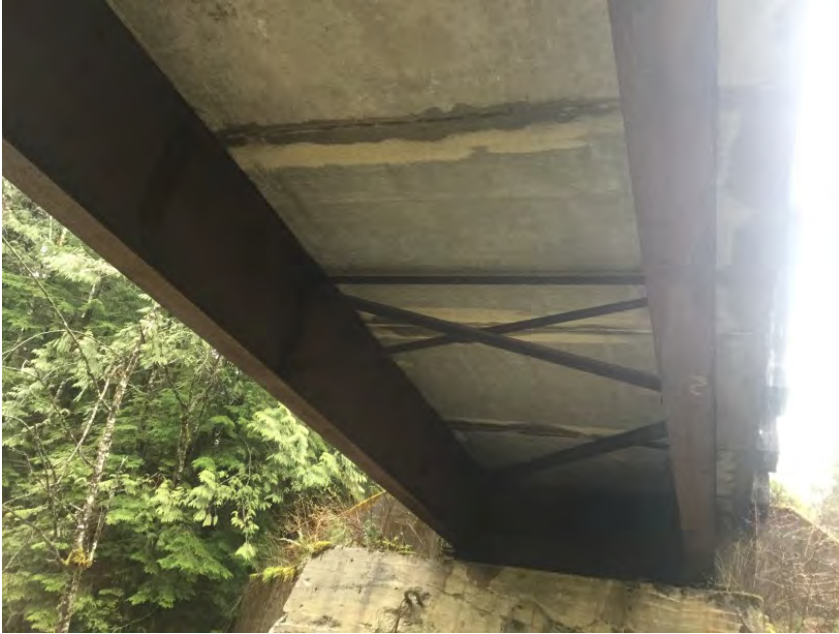
Jumpspan deck joints have evidence of water getting through
